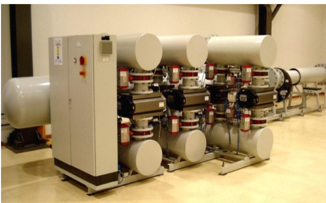
Fig. 2. TGS gas flow laboratory
