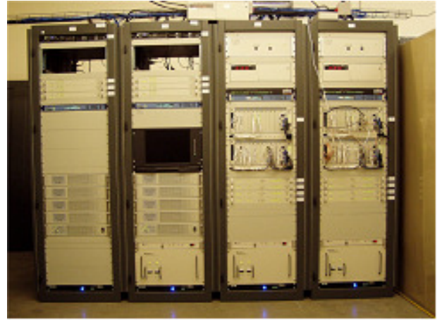
Figure 3: Photo of a 4 rack dual-redundant time-scale system that supports up to 6 local clocks and an unlimited number of remote clocks
