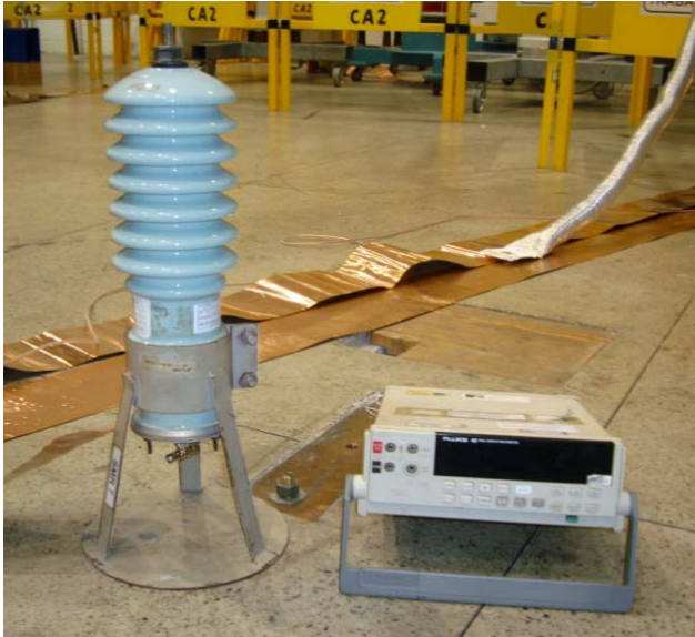
Figure 2. Photo of RMS7 to AC High Voltage.
