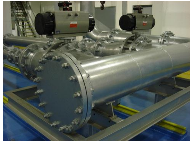
Fig. 9. Partial view of the test section highlighting the header for receiving oil from the test lines
