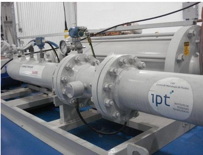
Fig. 11. Compact prover and turbine meter
